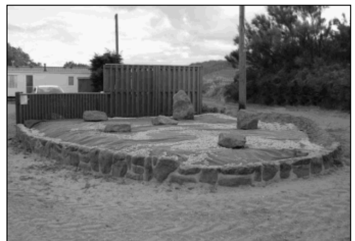
Work in progress - work underway on the new bed at North Beach. [photo by Rob Topliss]
